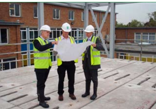
Starting work... Belvoir High headteacher, Jon Sherwin (left) and deputy head, Paul Ainsworth (right) with building manager, Terry Downes
