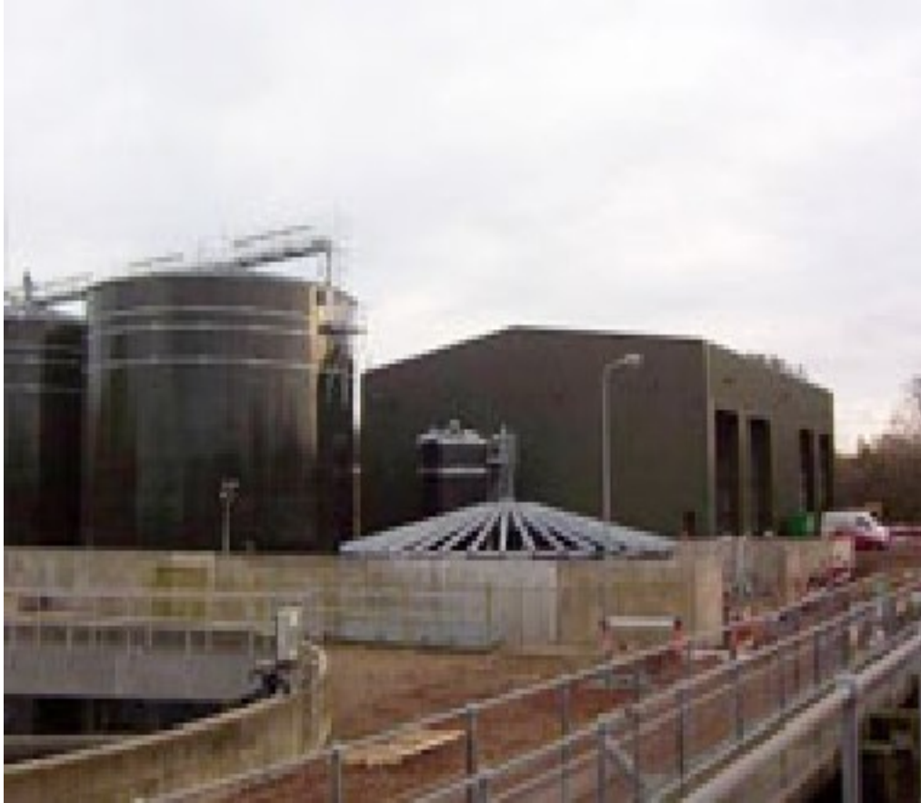
Biogas AD Plant, Warrington
